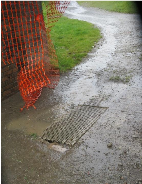
The likely cause of sinking bridge abutments
