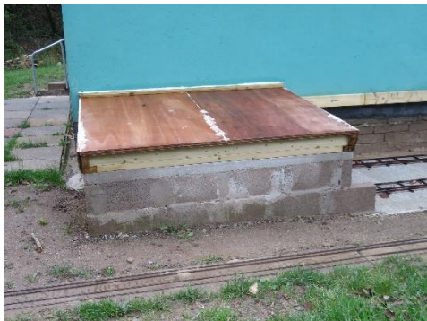
Improved protection for the electricity supply
