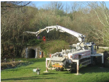
The pump ready
