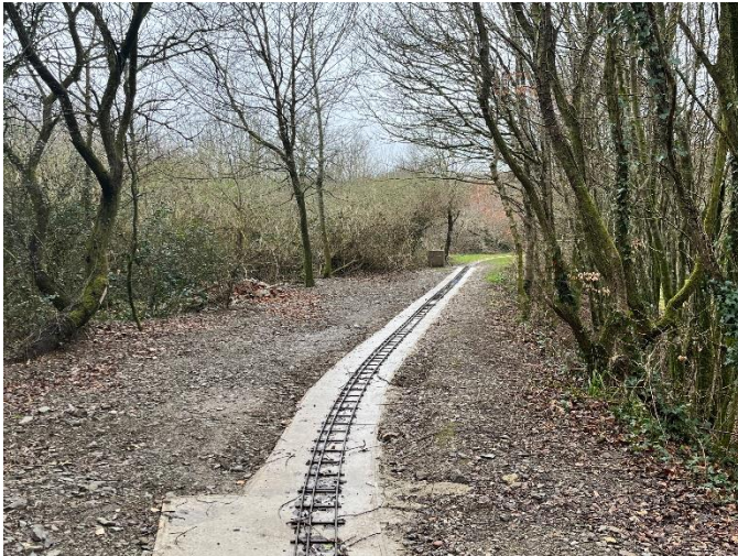
Looking up towards the bridge, newly laid track awaits top screed on 12 th March 2023.
